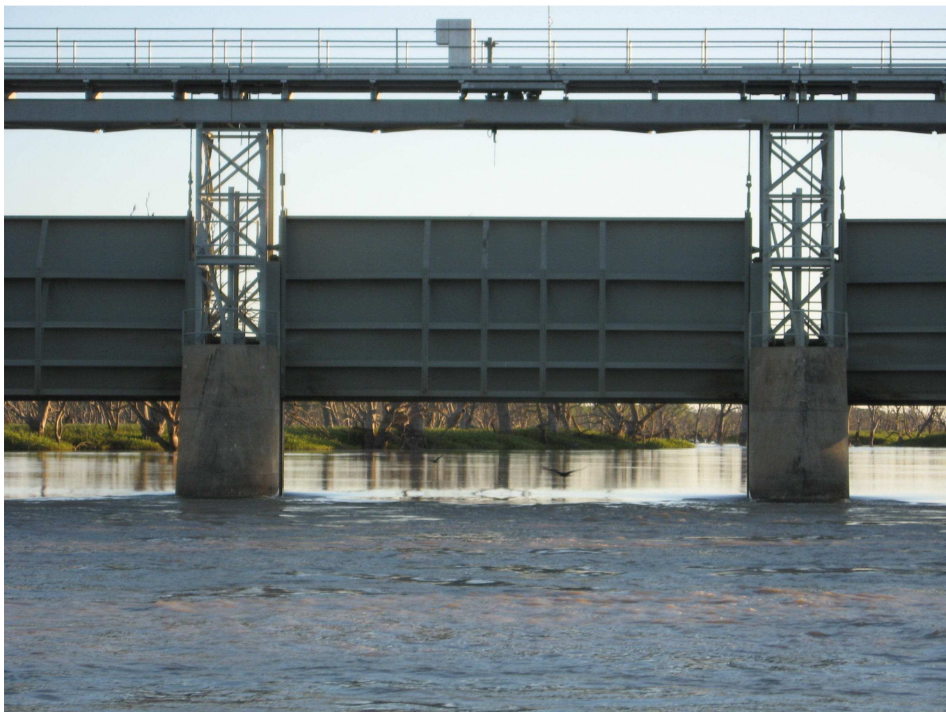
Menindee Main Weir gates looking upstream into Lake Wetherell – 12 March 2012 Courtesy Barry Philp, SWC
