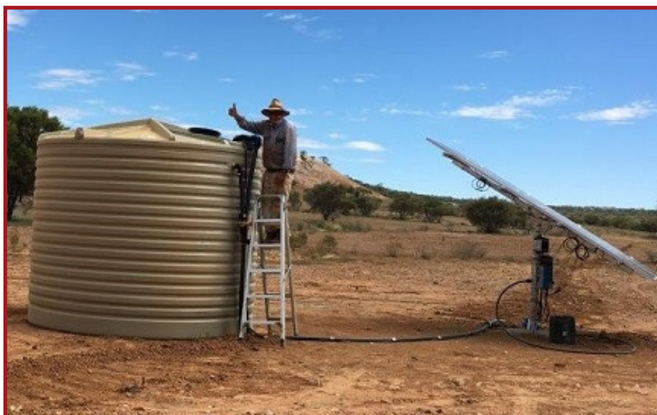
Above: Grant Cooney hooking up poly tanks and solar panels at Tarko .
